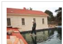
Spencer Brown Presidio Development Director Scott Ward tests a living roof under development.
